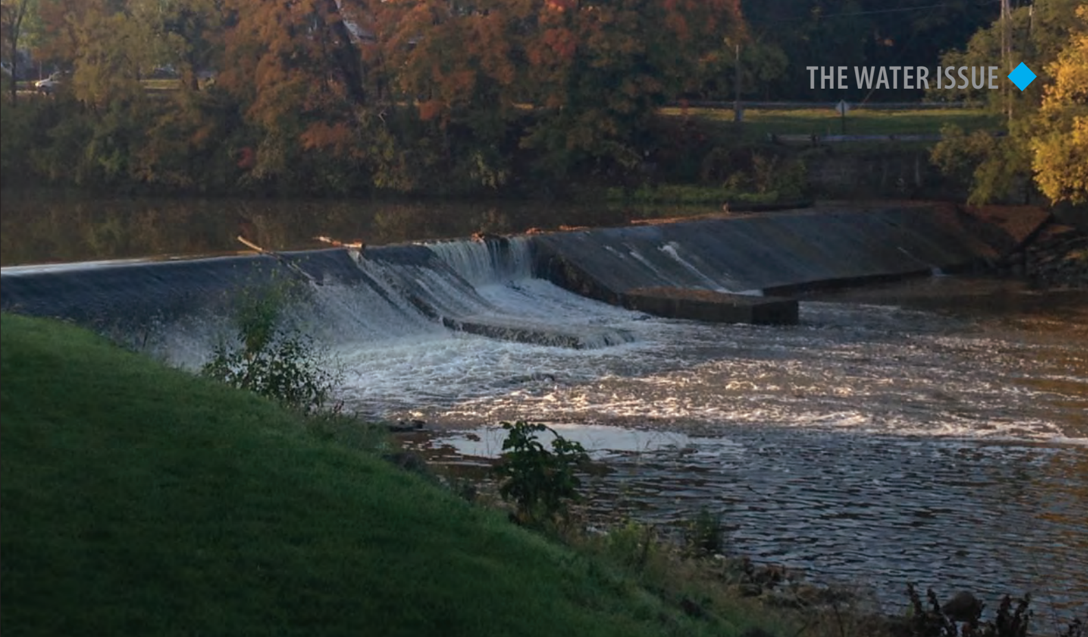
Built in 1850, the Cass River Dam was demolished as part of the Frankenmuth Fish Passage project. PHOTO BY MATTHEW MATTESON, CTI AND ASSOCIATES INC.
